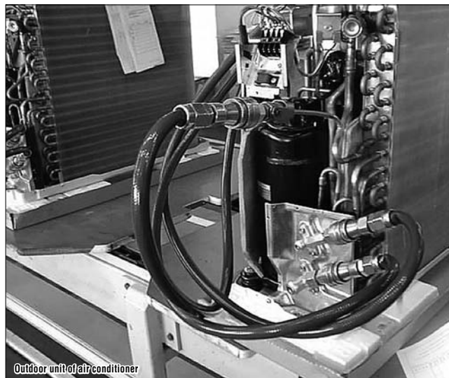
Outdoor unit of air conditioner
